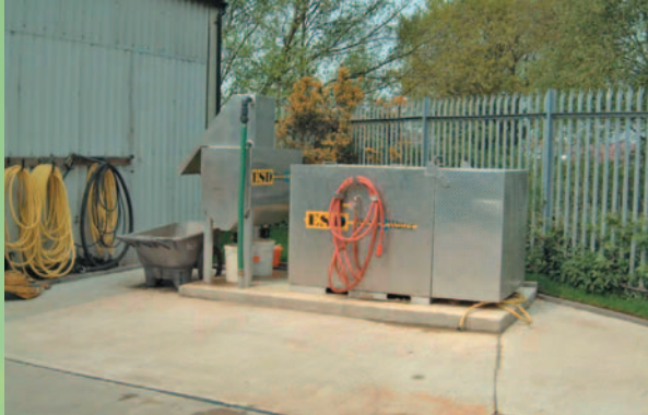
Groundsmen use a closed loop water system to wash machinery, reducing water usage.
